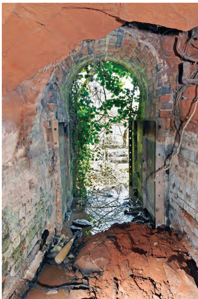
The iron frame of the waterwheel penstock. Note how tree roots are coming through the sandstone
